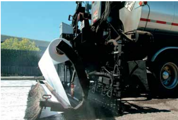
Mechanical installation of TruPave® on a sound substrate using a bitumen bond coat.
