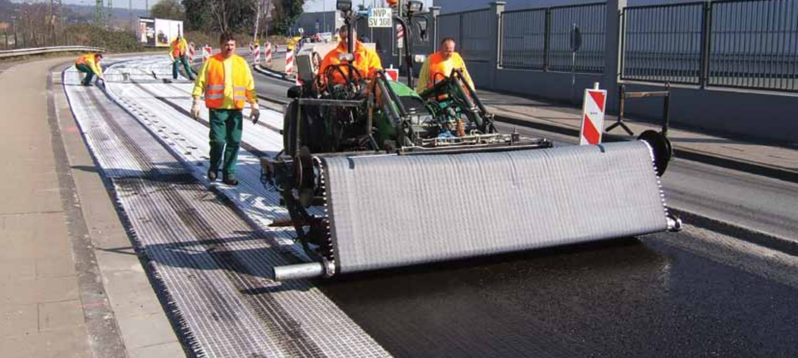
Mechanical installation of Tensar Glasstex® is fast and efficient – an experienced crew can install up to 12,000m 2 per day, per tanker.
