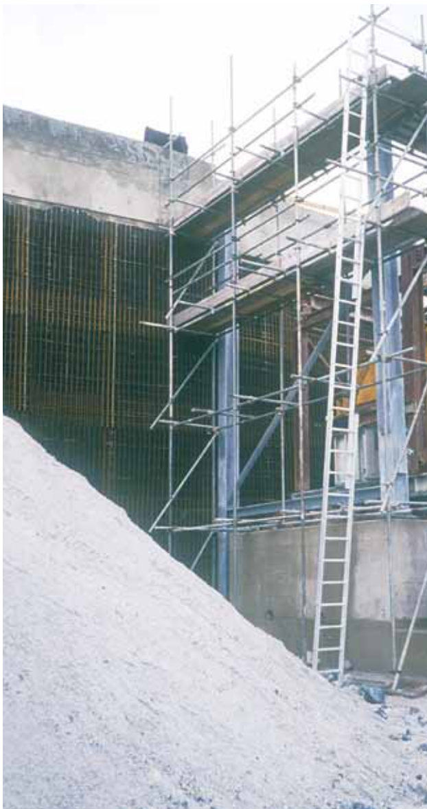
TensarTech TR2 steel mesh panel system at Lee Moor Crushing Plant offered considerable savings over a concrete faced alternative.
